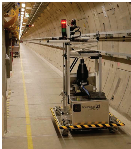
Figure 2: The current appearance of MARWIN in the XFEL tunnel
